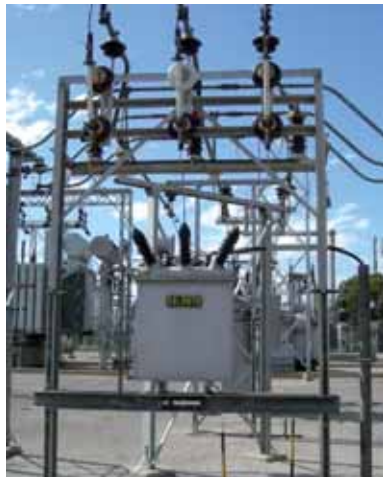
A 22kV Station Service Transformer
