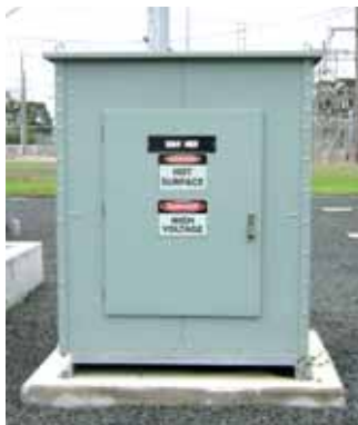
A 22kV Neutral Earth Resistor
