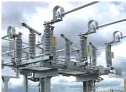
66kV ganged rotary isolator
