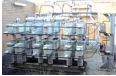
A 22kV Capacitor Bank
