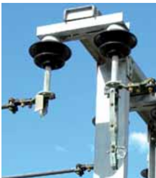
22kV Single phase isolator
