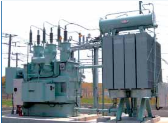
A 66/22kV transformer with separate oil cooling arrangement
