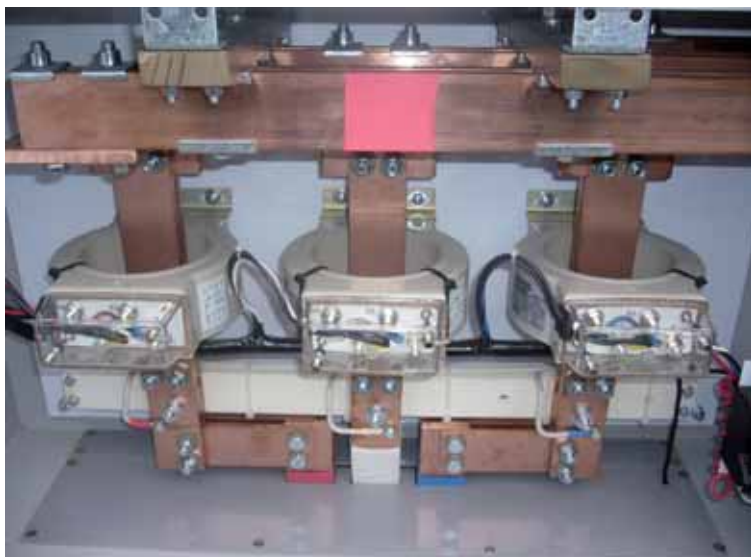
CT Chamber showing LV buswork and CT's
