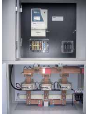
CT Metering enclosure showing meters and separate CT Chamber
