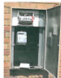
Main Switchboard/Metering Enclosure
